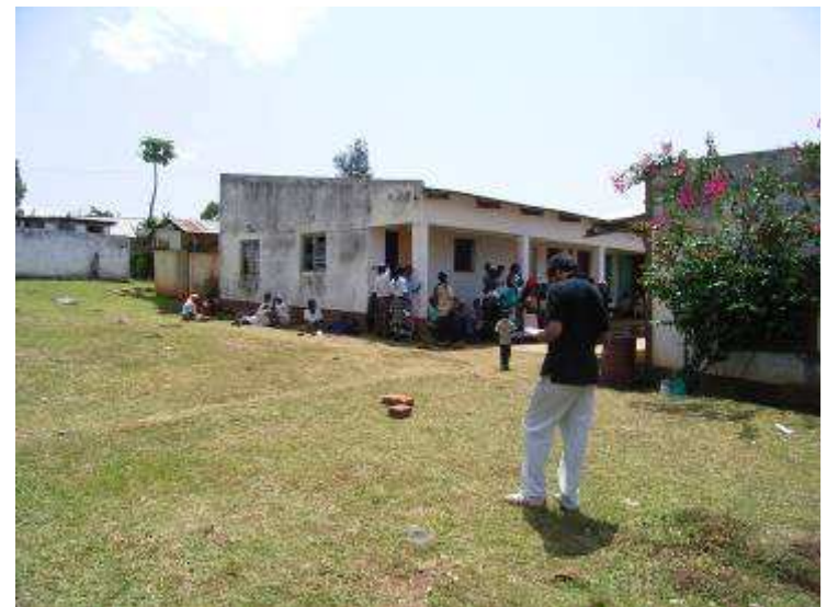
The building and its roof to be fixed in future
